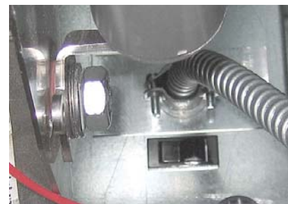
Figure 14 (Rear view of Control Box)
