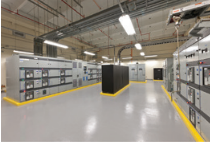
Figure 1. MCCBs protecting critical equipment at the Eaton Bluegrass Data Center in Bluegrass, KY.
