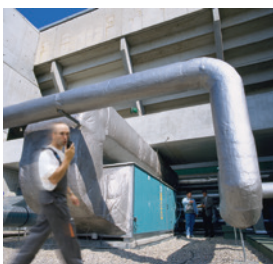
Air handling unit
